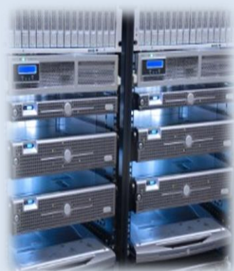
GuestLinX data center is powered by Dell Servers
